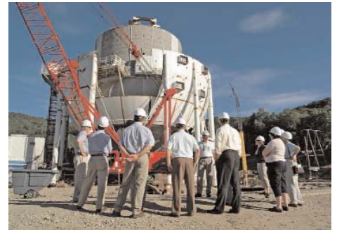
Members of the Yankee Rowe Community Advisory Board (CAB) - which has been meeting since 1998 to monitor decommissioning - toured the Yankee Rowe plant on June 16, 2004 prior to their most recent meeting. Above: CAB members view the progress of the dismantlement of the large white containment sphere.
